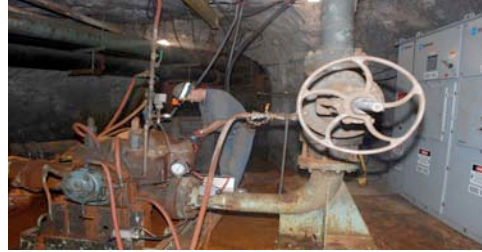
Sanford Lab Infrastructure Technician Bill Heisinger, a former Homestake miner, adjusts a 700-horsepower pump on the 3650 Level at Homestake
