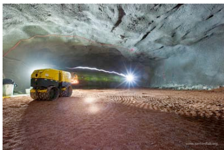
Figure 3: Transition Cavern of Davis Campus 4850 Level, seen here during outfitting, excavated in 2010. Now home to the MAJORANA DEMONSTRATOR experiment
