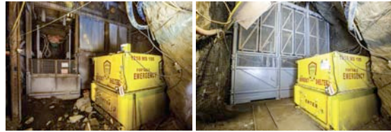
Figure 8: The 1250 Level station rehabilitation - Before and after (The yellow box is an emergency shelter).
