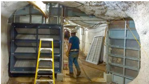
Figure 5: Terry Garcia of Ainsworth-Benning Construction in the newly-constructed Kennedy drive-through structure (right). The filter system (left) is designed to keep the air in the copper electroforming lab clean. Fan is on the back of the filter wall.
