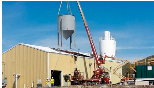
Figure 6: The new tank is lowered through the roof of the influent building
